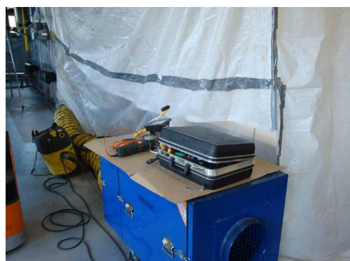
Fig. 3: Negative pressure enclosure – air cleaner with HEPA filter
